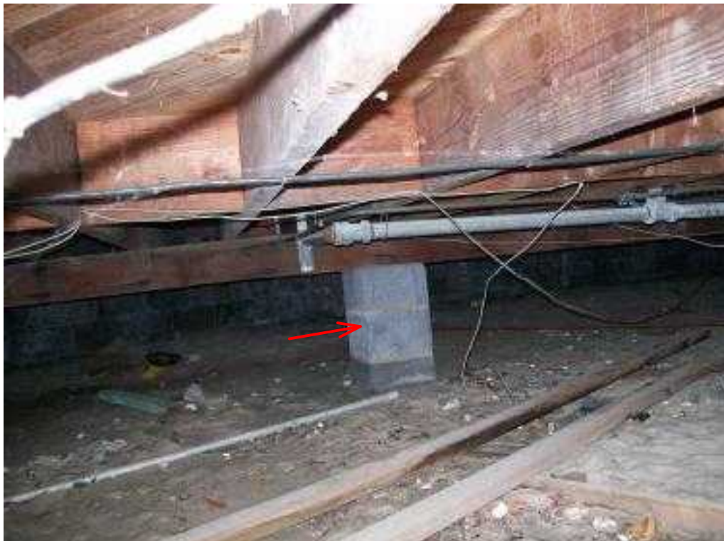
Single block pier for supporting main beam approximately 45 lf. Pie footings should be placed approximately every 72" center to center. Galvanized drain lines in an unconditioned space.
