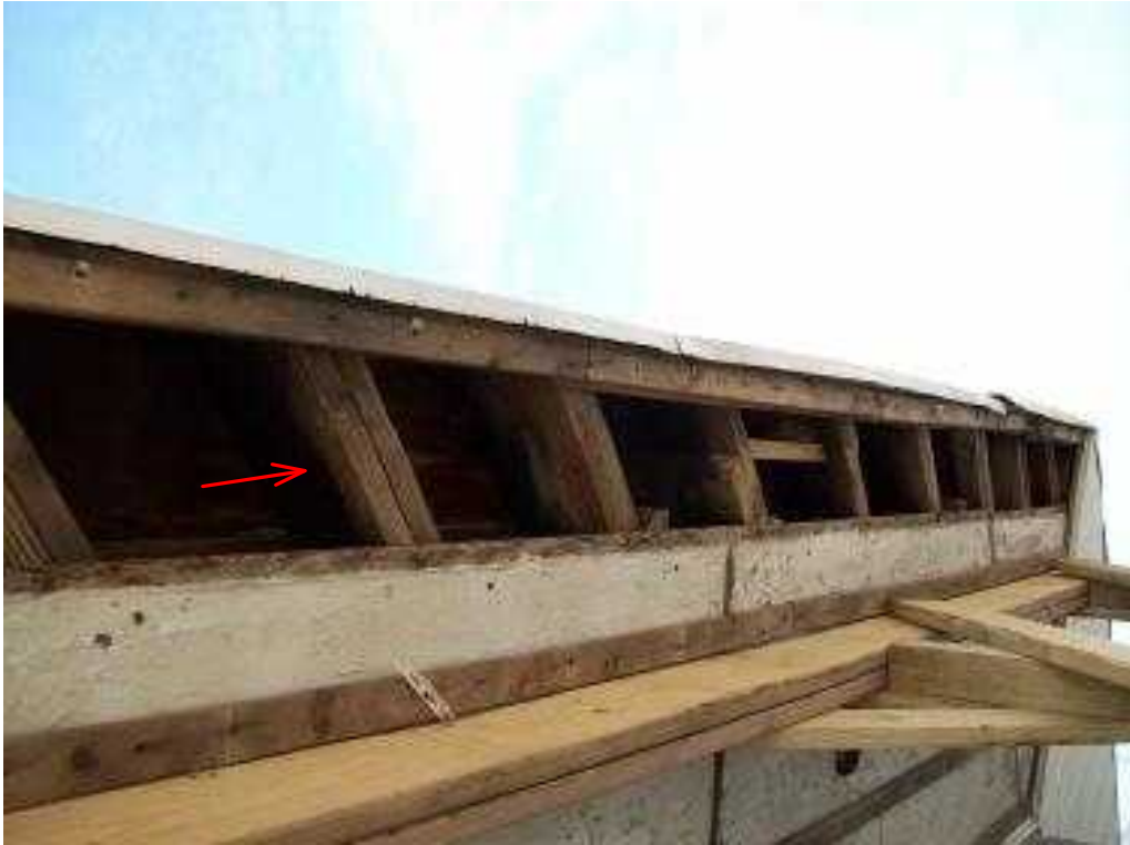
Undersized balcony framing and the beam projection into the building should be 3 x the length of the projection, existing condition does not meet this criteria.
