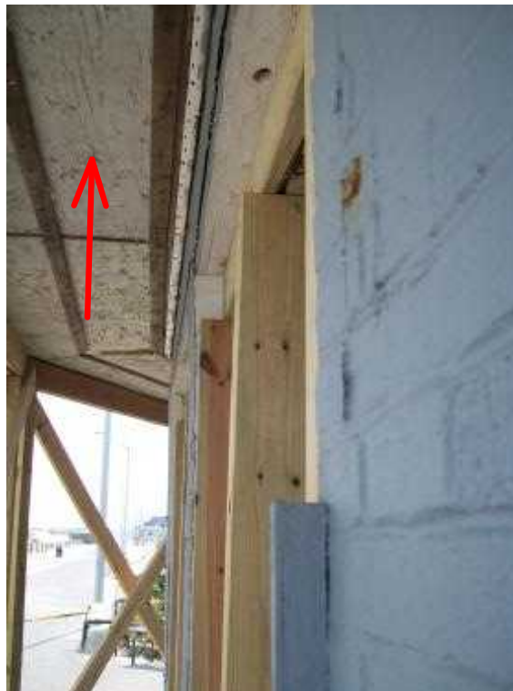
Unvented soffit moisture damage to plywood.
