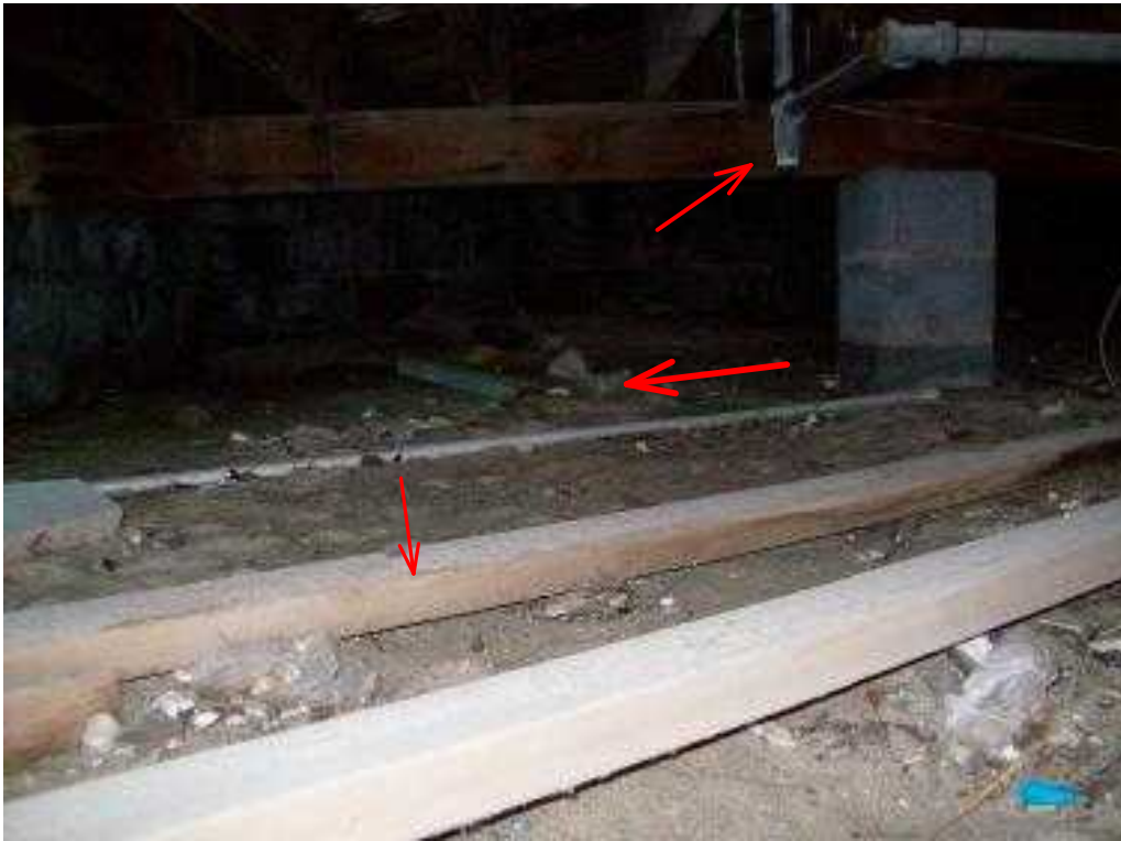
Foundation floor has no vapor barrier causing moisture damage to the floor beams, girder and piping systems
