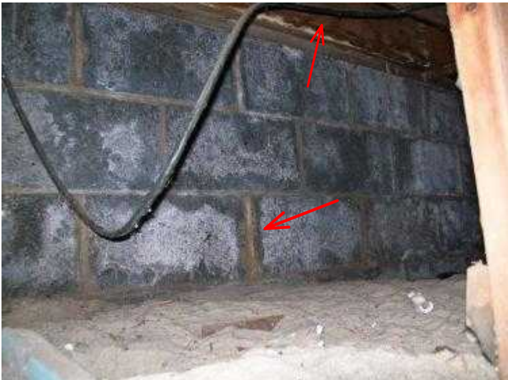
Continued moisture damage.
