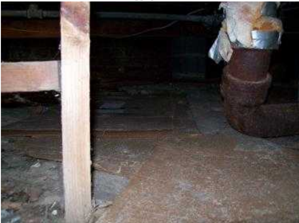
Damage plumbing with more temporary supporting.
