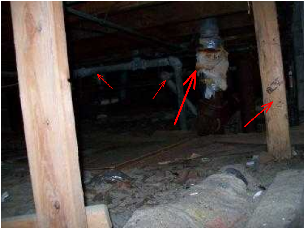
Continue moisture damage to components in crawl space. There many temporary supports in place.
