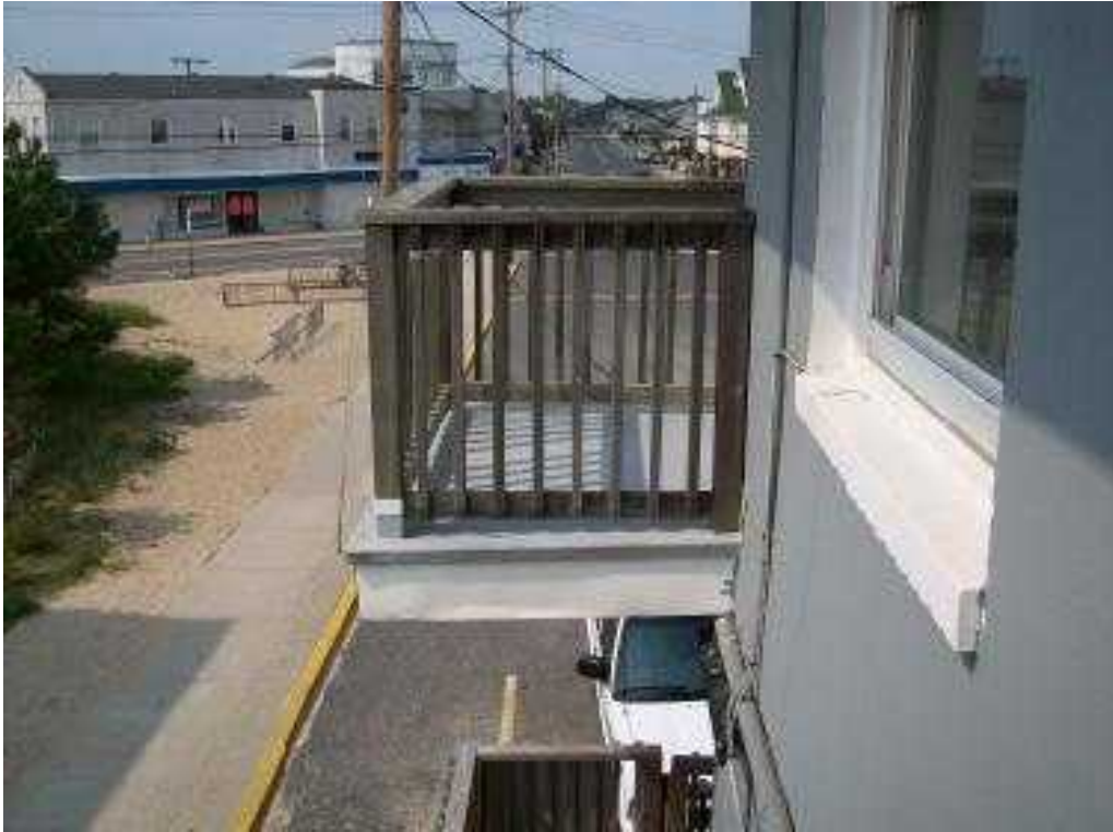
Balcony leaning due to non compliant framing system.
