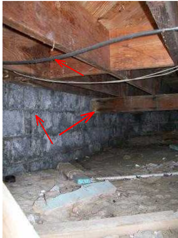
Additional moisture damage.
