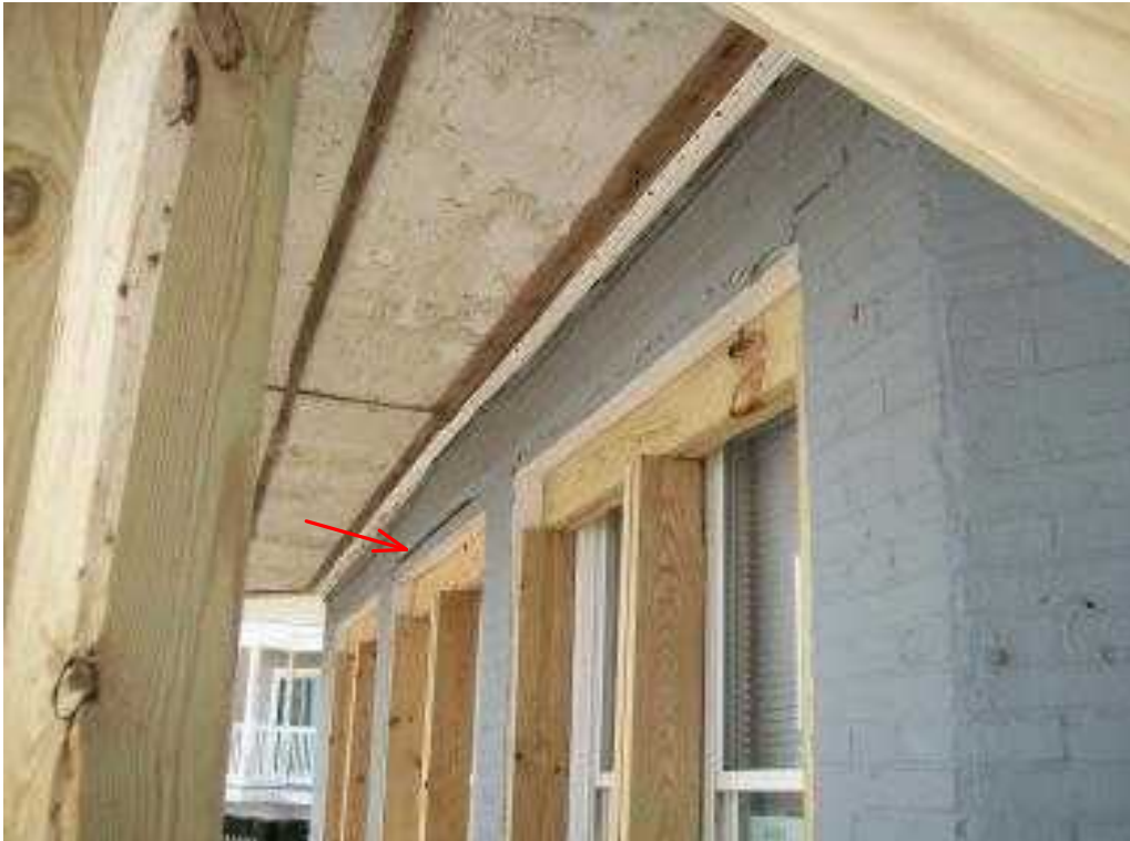
All lintel supports dry rotted require replacement.
