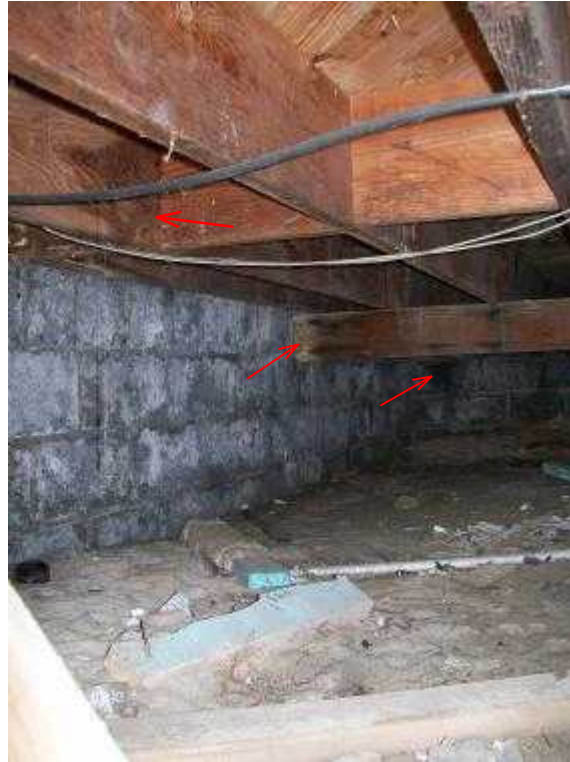
Main beam undersized dry rotted where it pockets into block wall with no additional support base. The beam is undersized for the live load of this building. Water staining on every component.
