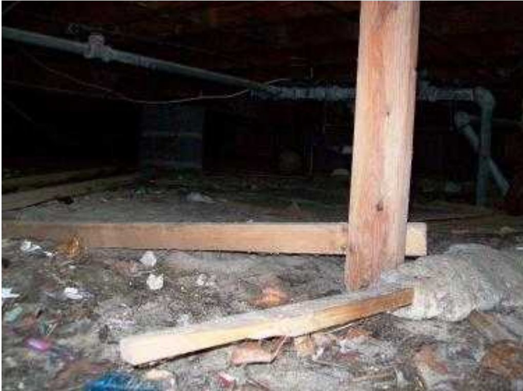
Galvanized water lines, outdated rust from interior of pipe slowing water pressure to the supply areas.
