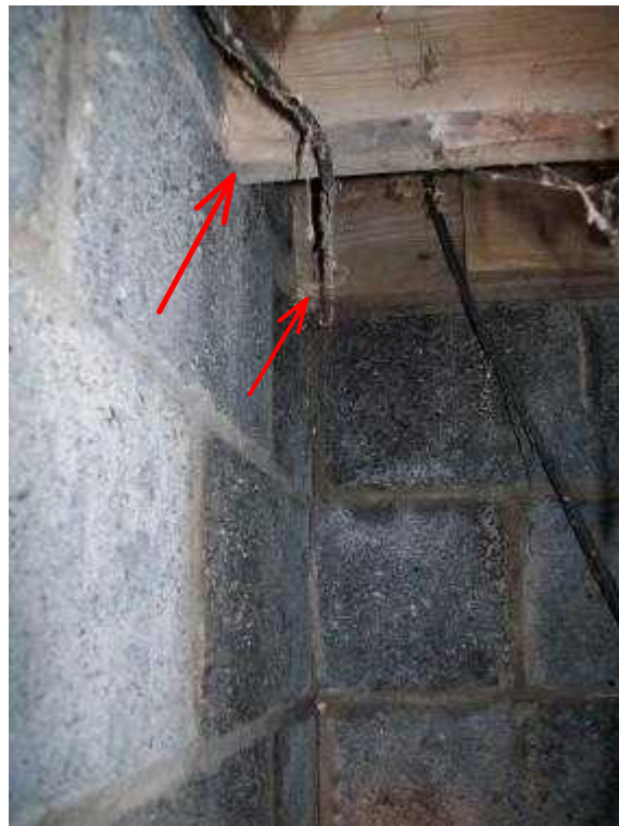
Floor beams damage at bearing points by moisture due to unconditioned space.
