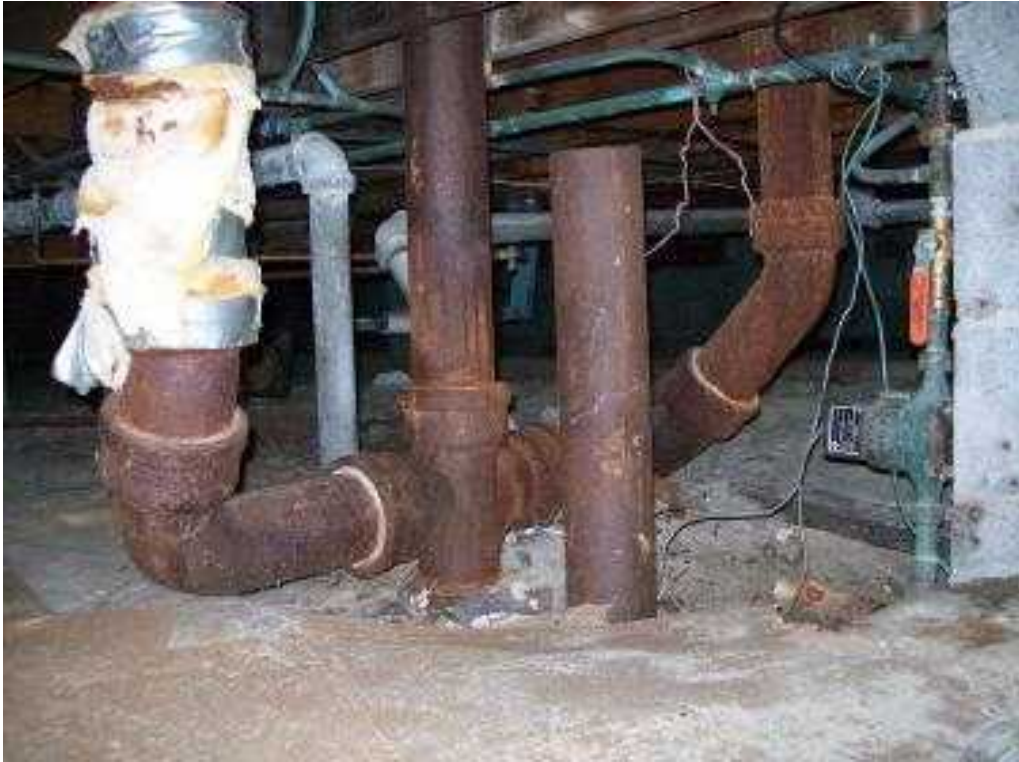
Out dated plumbing system all piping shows signs of moisture damage.
