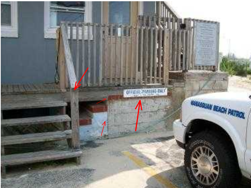
Handyman style deck construction not code compliant.
