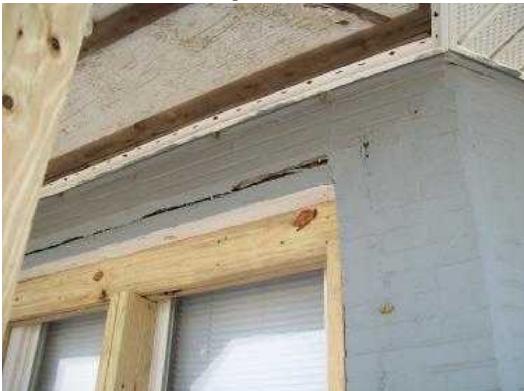
Dry rotted lintel system, requires replacement.
