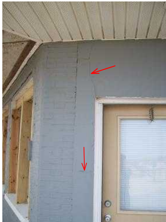
Walls were filled in between piers without expansion process causing stress cracks.
