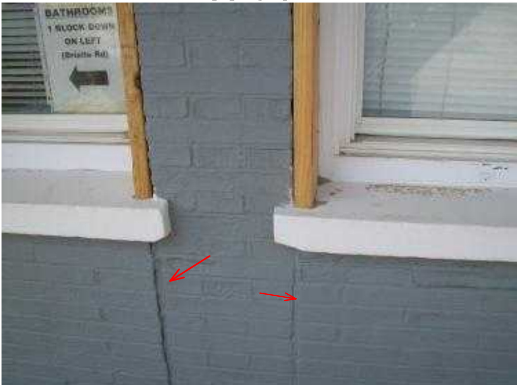
Wall fill in no expansion. The wall is moving outwards because there is no connection to the pier and expansion is not in place.
